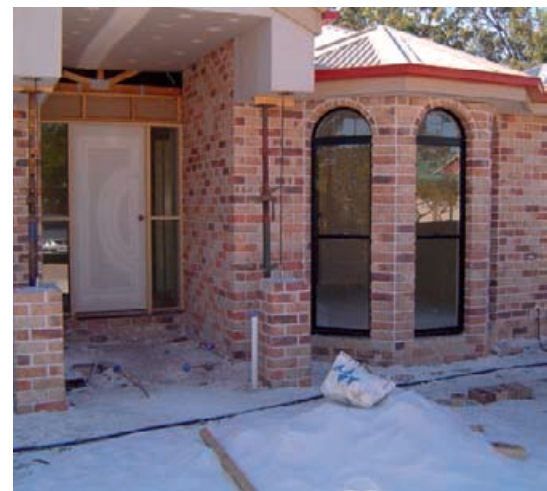
The style and colour of clay bricks creates a beautiful contrast with the pure white cement mortar.
