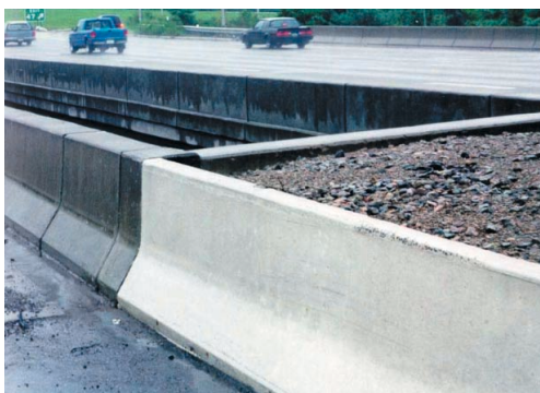
New Jersey Barriers are often made of grey concrete.
